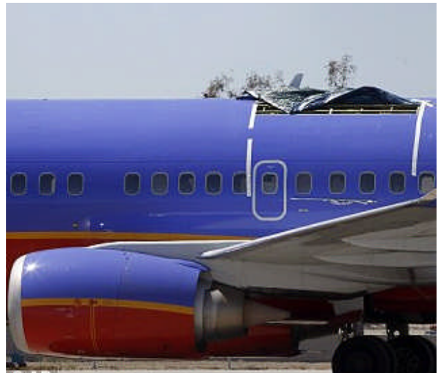
Figure 11 Tarpaulin covering the five-foot-hole that ripped open in the roof, from [16].
