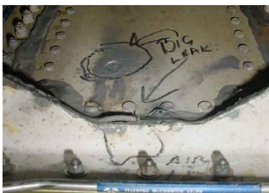
Figure 3.2.3 Photograph of bulkhead fastener leakage area.
