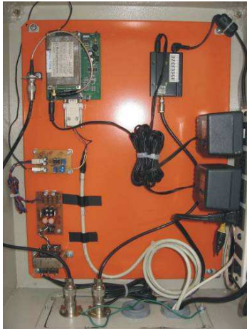
Fig. 15. Equipments on the tower
