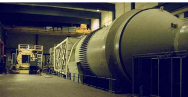
Fig. 7: T-38 hall. T-38 is a blowdown-type wind tunnel with 1.5 x 1.5 m and 0.38 x 1.5 m test sections and trisonic Mach number range (0.2 to 4). It is driven by air stored in 2600 m 3 tanks charged to 20 bars pressure by a 4 MW compressor.
