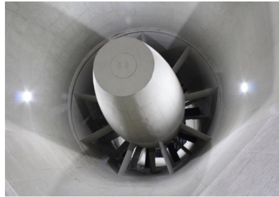
Fig.7 Photos of the fan during testing phase
