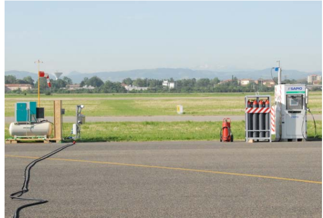
Fig. 20 – APL S100 Refuelling System
